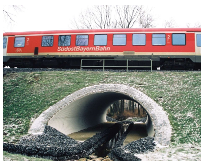
Picture 5: Culvert with double sidewalk for amphibians, small animals, etc.
